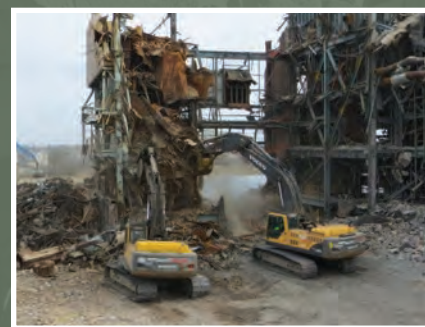
NADC contracted for complete abatement and demo of the National Grid Far Rockaway power plant.
